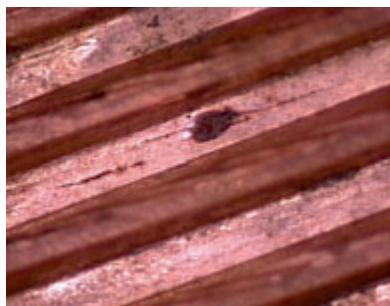
Figure 3. Corrosion Pit in Grooved Copper Tube (Photo Courtesy of Corrosion Testing Laboratories, Inc.)[1].
