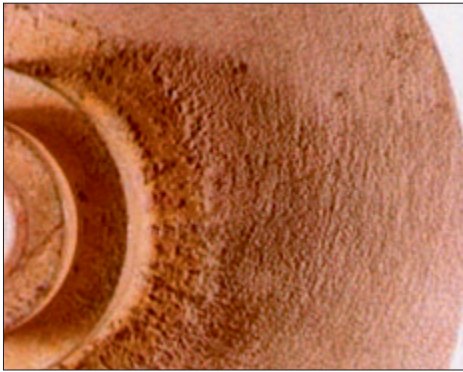
Figure 8. Erosion (Cavitation) Corrosion of a Brass Pump Impeller. Air Bubbles Eroded the Soft Copper Oxide Protective Layer Enabling Corrosion of the Base Metal. (Photo Courtesy of Corrosion Testing Laboratories, Inc.)[1].
